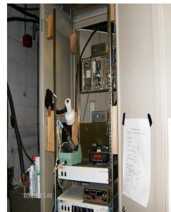
Starting from top. Receiver for north link with cover removed. Receiver main site cover attached. Digital voice recorder, with Yaesu control receiver and soldering iron sitting on top. ACC controller with digital volt meter sitting on top. A paper with some notes and commands is taped to door.
