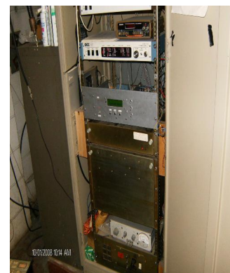
From top, bottom half of cabinet. ACC repeater controller.
